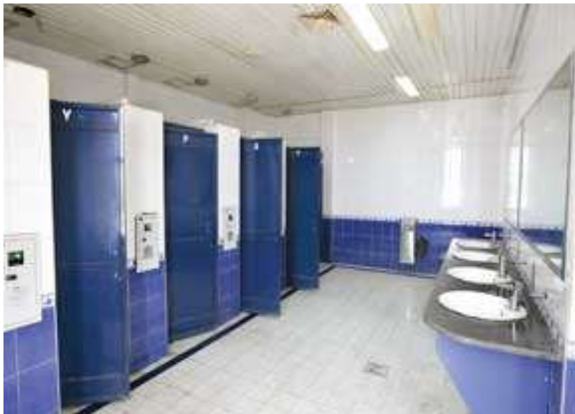
Fig. 5. A view of a sanitary service with good conditions
